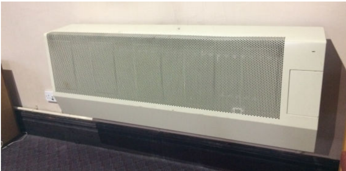
Photograph 2: Church Gas Heaters
