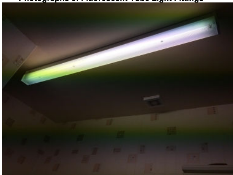
Photographs 8: Fluorescent Tube Light Fittings
